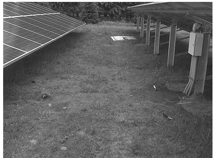
Fig. 5. Site showing the initiation of bare ground below the panels, which increases the potential for erosion (photo by John Showler, reprinted with permission)
